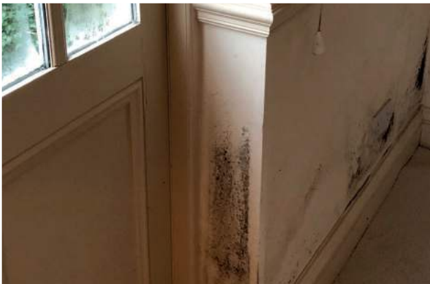
Mould and condensation problems around window reveals and corners
