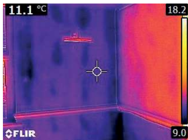
IR image captured part way through application. The left-hand wall has not yet been treated and is cool with dramatic cold bridges (purple blotches). The SprayCork treated right-hand wall is much warmer and the cold are eliminated (solid orange / red)
