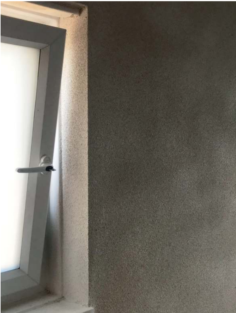
The granular CorkSol layer, spray-applied seamlessly including round the window reveal, ready to accept the final plaster skim.
