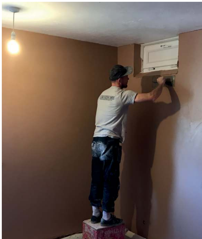
The Good Plastering Company apply the final plaster skim, leaving the room only 8mm smaller.
