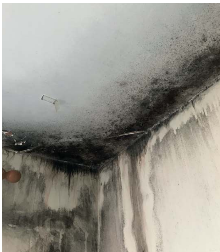
The most severe patch of black spot mould, just before the remedial work began.
