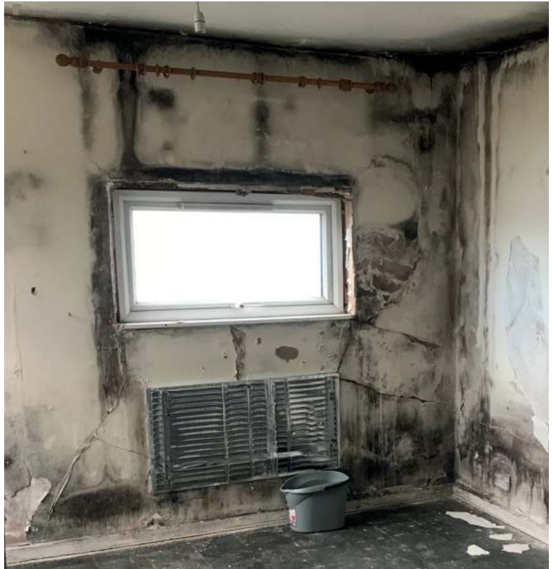
Black mould is rife in the flats, but especially at ceiling and floor level and around the window reveals.
